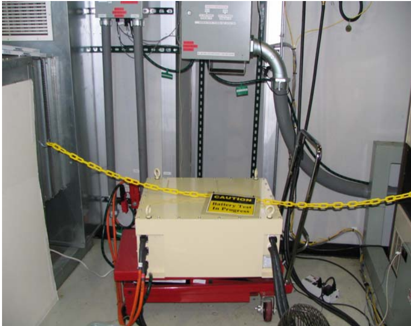
Real Battery – SAFT VL41M
